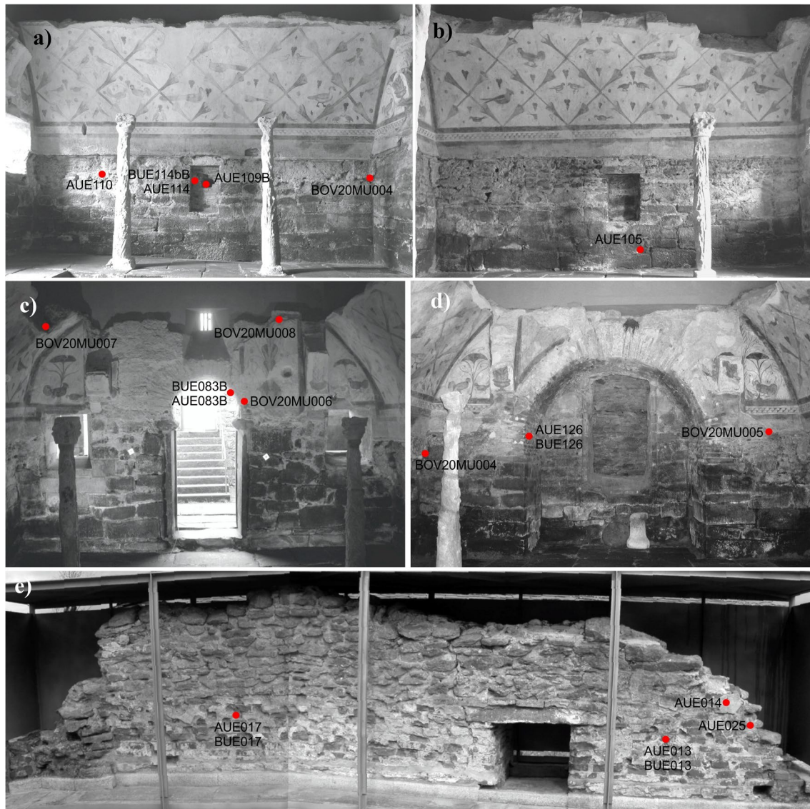
Fig. 3 Samples' location. a North wall of the aula. b South wall of the aula. c East wall of the aula. d West wall of the aula. e Remains of the vault of the upper floor
